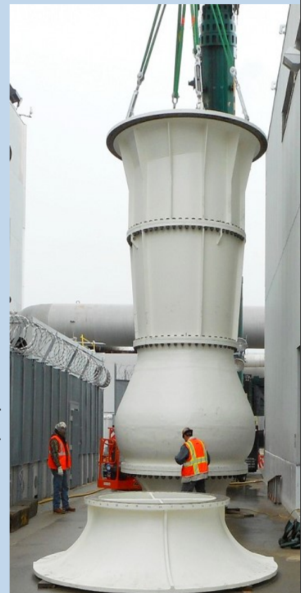
AFTER BEING ASSEMBLED OUTSIDE PUMP IS BEING LIFTED TO INSTALL IN PUMP BASIN
