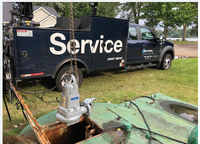
Flygt Concertor's discharge design allowed it to be installed with the existing manufacturer's guide rail bracket.
