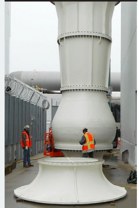
After being assembled outside pump is being lifted to install in pump basin
