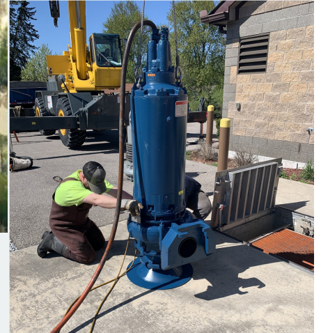
Thomas Township needed to pull, repair, and reinstall one of their four main 100 HP Weir Specialty Submersible Pumps.
