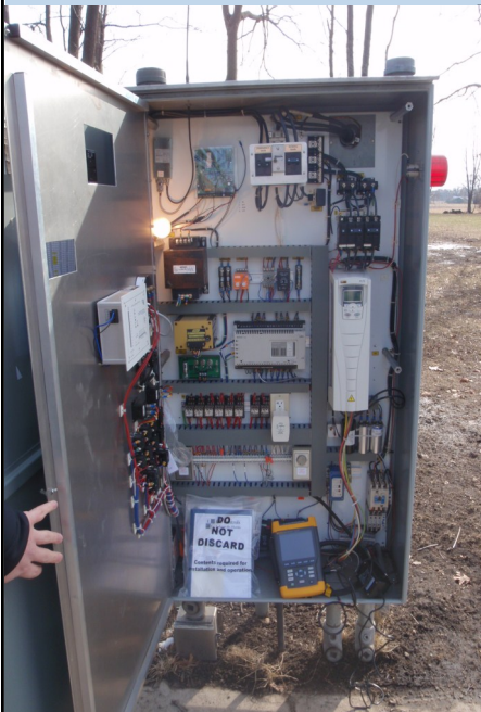
Control panel with VFD for phase conversion
