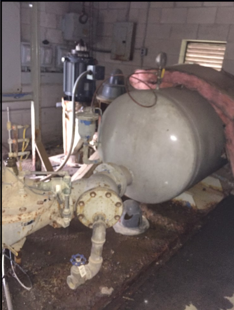
FAILED ORIGINAL PUMP SYSTEM
