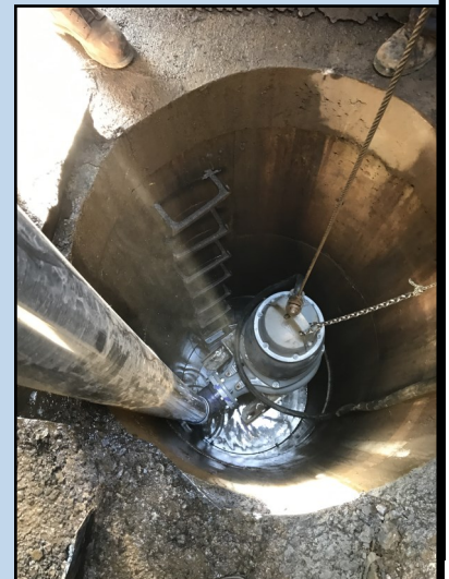
NEW PUMP IN WET WELL
